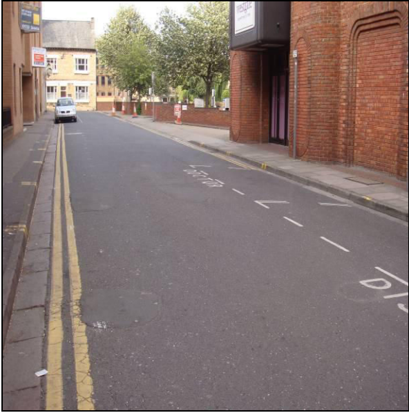
Figure 1 North Street before Resurfacing
