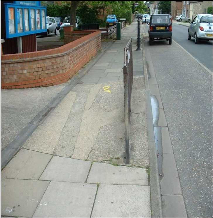
Figure 9 Footway in Church Street, Werrington before Slab Replacement
