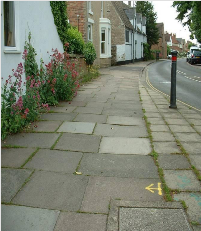
Figure 17 Church Street Werrington before Slab Replacement Scheme
